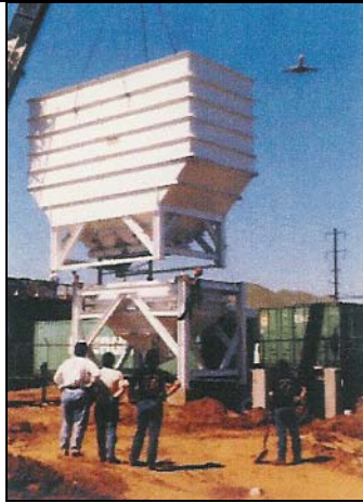
From Foundation to Electrical Wiring and from Mechanical Erection to Full Enclosures
